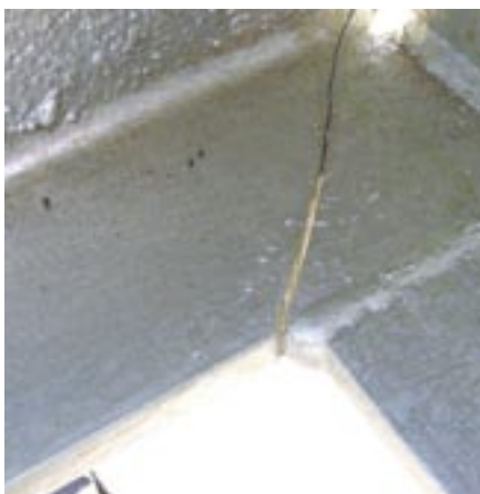
Suspected LMAC defect in angle frame with crack propagation from welded corner.
