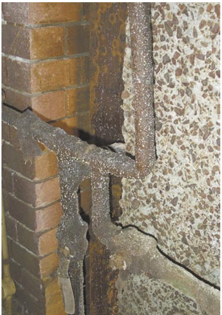
This gas pipe junction was petrolatum tape wrapped in 1978 and remains in good condition in 2005 in a very aggressive environment, as indicated by the condition of the steel and concrete.
