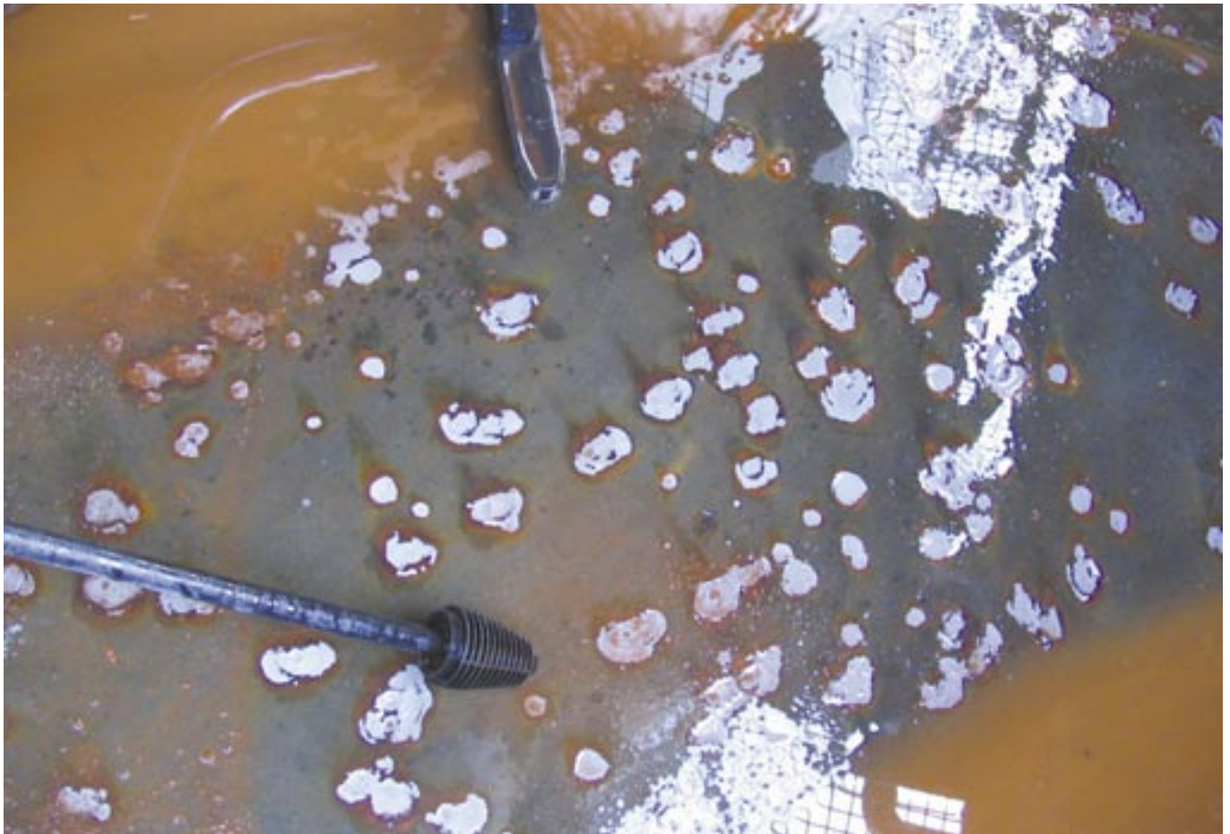
The white areas are steel that has been 'pickled' by acidic microbiological excretions in a cooling water tank. MIC has corroded over 1 mm of steel in less than 2 years.
