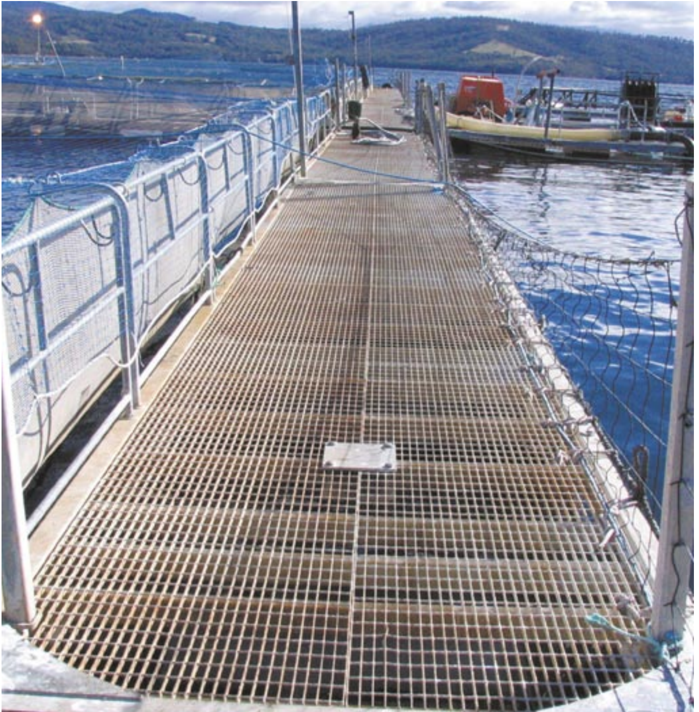
Marine exposure – salmon farm pens in southern Tasmania. High corrosion rate of the galvanized steel in the splash zone on these structures limits coating life to less than 10 years in this type of water.
