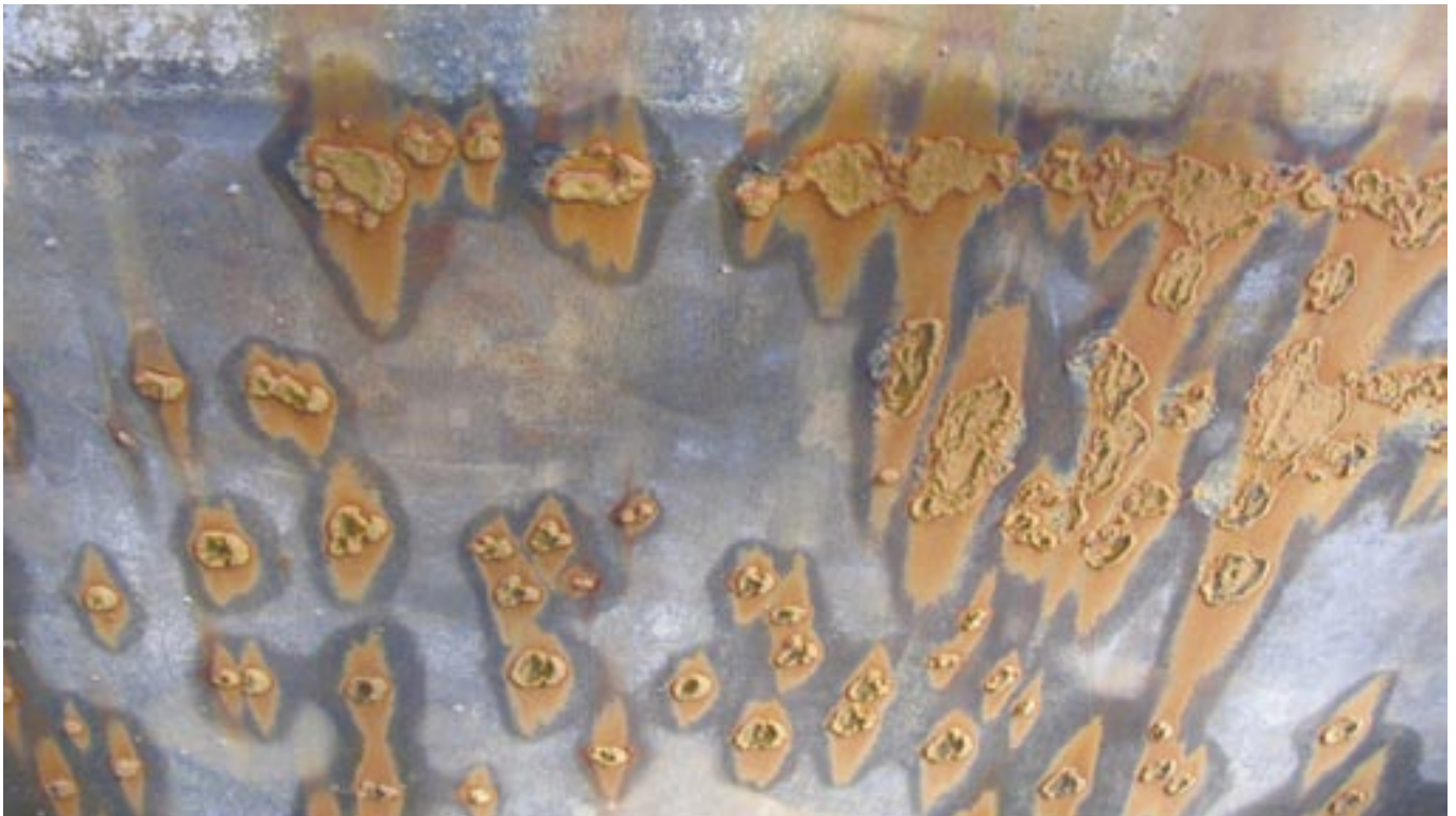
These corrosion nodules have formed on a galvanized cooling water tank and are typical of microbiological corrosion. The water treatment additives in this system have contributed to the accelerated MIC activity.
