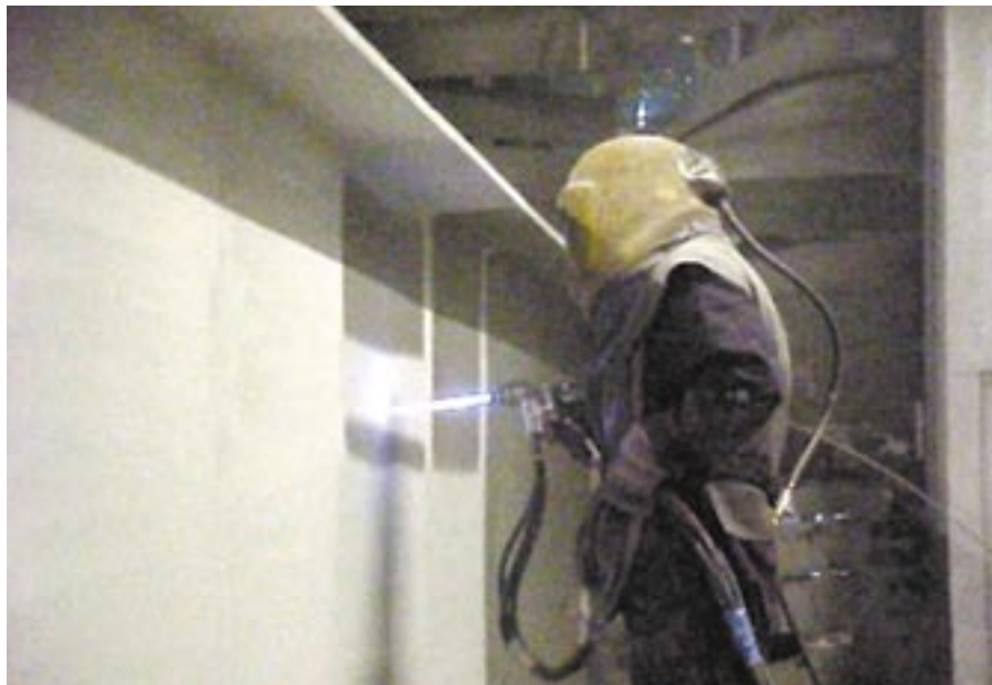
Zinc metal spraying of large structural sections is a cost effective method of applying a metallic zinc coating to steelwork too large to galvanize.
